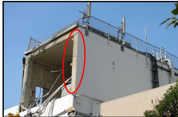
Precast concrete wall panel connections failure at a local telecom hub damaged HVAC system at this critical facility.
