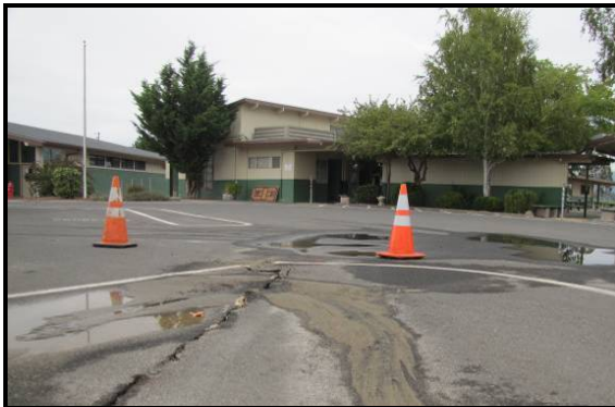
Ground rupture in an elementary school parking lot south of Napa resulted in fracture of underground water piping.
