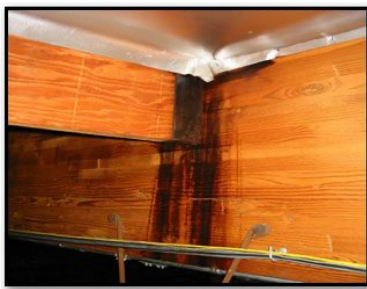
Dark Streaking on Purlin Hangers
