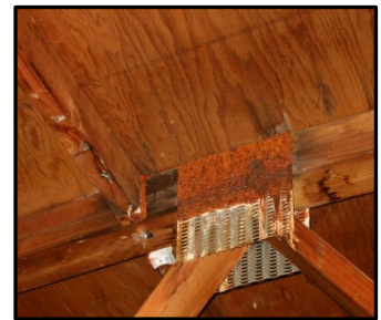
Rusting Gang Nail Plates
