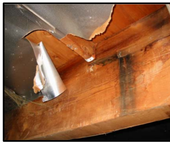
Discolored/Sagging Sub-Purlin Hangers
