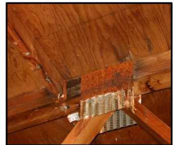
Rusting Gang Nail Plates
