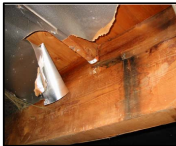
Discolored/Sagging Sub-Purlin Hangers
