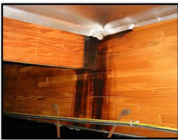
Dark Streaking on Purlin Hangers
