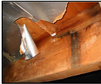
Discolored/Sagging Sub-Purlin Hangers
