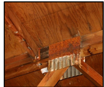
Rusting Gang Nail Plates
