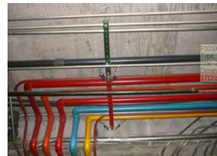
Equipment anchoring safeguards both business operations and building integrity.
