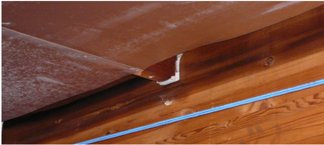
Notice the white corrosion formed on the sub purlin hanger
