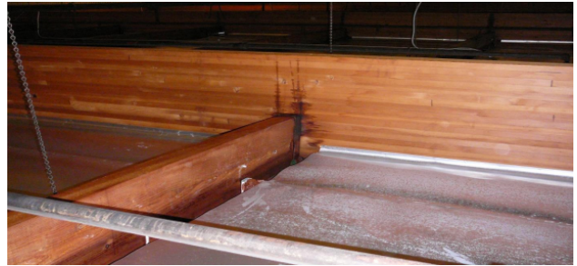
Notice the rusting of the purlin hanger from condensation
