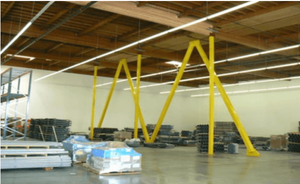
Large brace frame connected to a roof drag line for force distribution.
